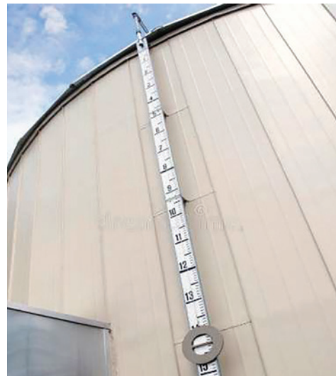
Figure 26: Example of a Tank Gauging System
